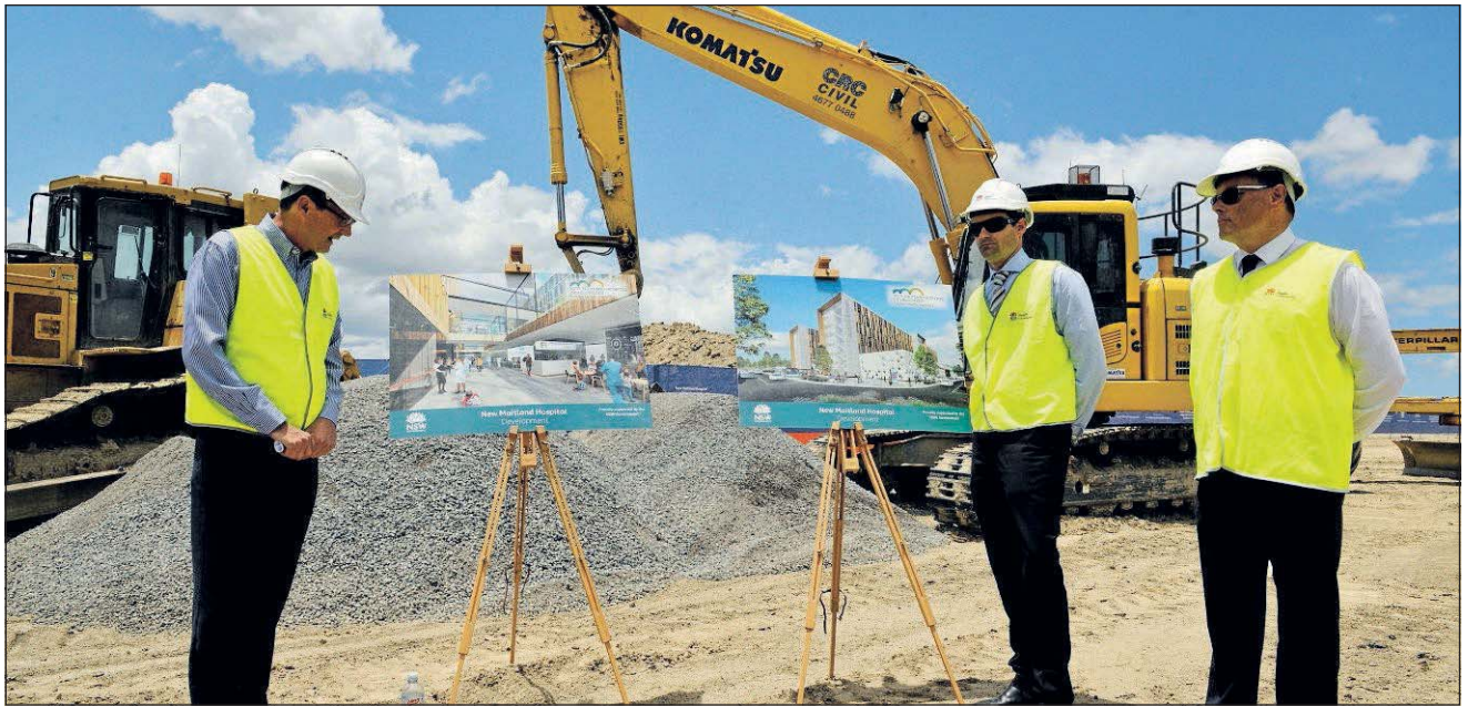
UNDERWAY: Scot MacDonald (left) unveils the new Maitland Hospital site last week with project director Gavin Thompson and New England health executive leader Eddie Pirillo. Picture: Lachlan Leeming
